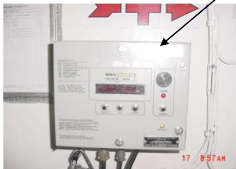
DIGITAL ALARM PANEL
