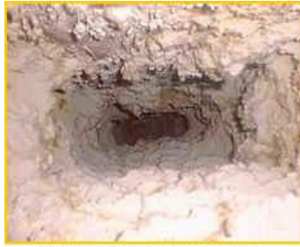
Buildup of dirt obstructs airflow through ventilation system
