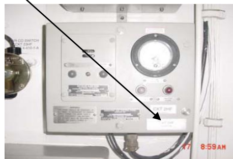
ANALOG ALARM PANEL
