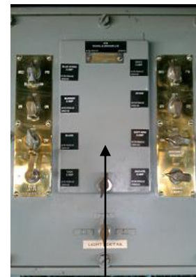
SIGNAL AND TASK LIGHTING PANEL
