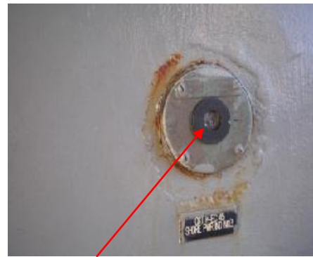
BROKEN INDICATING LIGHT LENS
