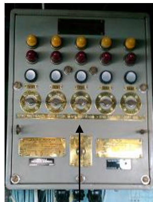
NAVIGATION LIGHTING TELLTALE PANEL
