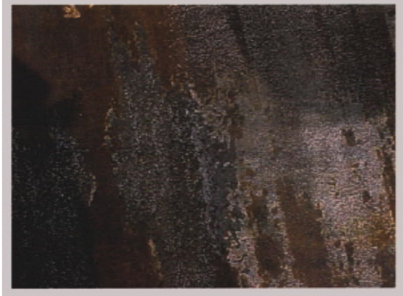
Figure 634-3-7. POOR SURFACE PREPARATION
