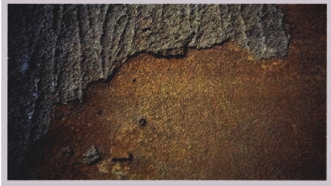
Figure 634-3-12. IMPROPER NONSKID APPLICATION
